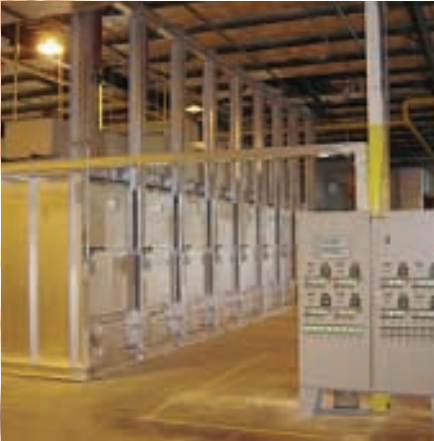
Thermal treatment at Wartburg/TN
